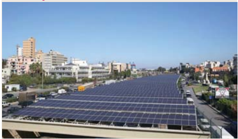
Photovoltaic panels are seen above the river bed in the Lebanese capital Beirut, yesterday. As part of the government's National Energy Efficiency Action Plan to instal 200 MW of solar farms by 2020, the construction of the Beirut River Solar Snake project is the largest of its kind on a national level.
