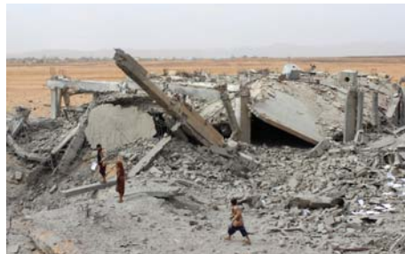
People walk on the collapsed roof of the Teaching Faculty after coalition air strikes destroyed it in Yemen's northwestern city of Saada, yesterday.
