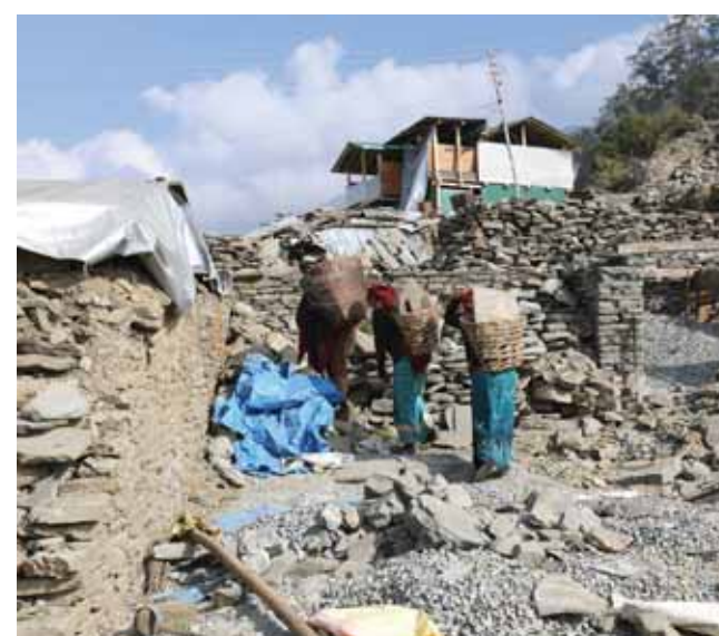
Local workers carry stones for building house in Barpak of Nepal's Gorkha district. Barpak, a village situated in the northern part of Gorkha district of Nepal, was the epicenter of the devastating earthquake that erupted on April 25.
